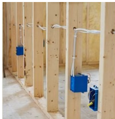
New Electrical Service
